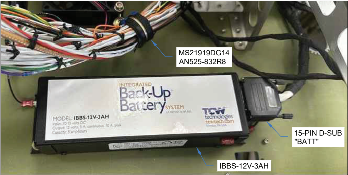
FIGURE 1: CONNECTING THE BACK-UP BATTERY
